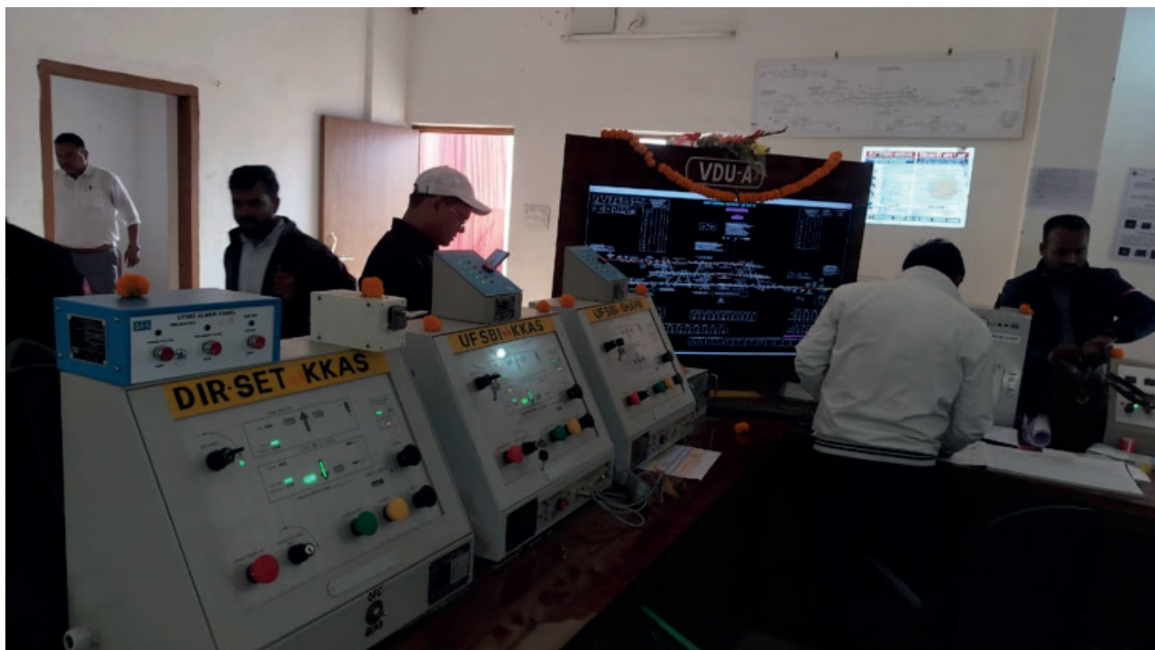
VDU/PANEL ROOM AT KATHAUTIA STATION
