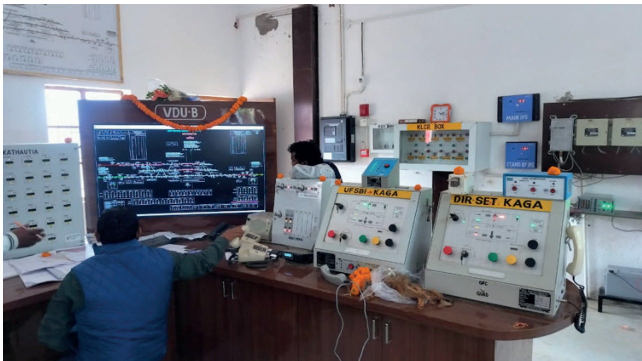
VDU/PANEL ROOM AT KATHAUTIA STATION
