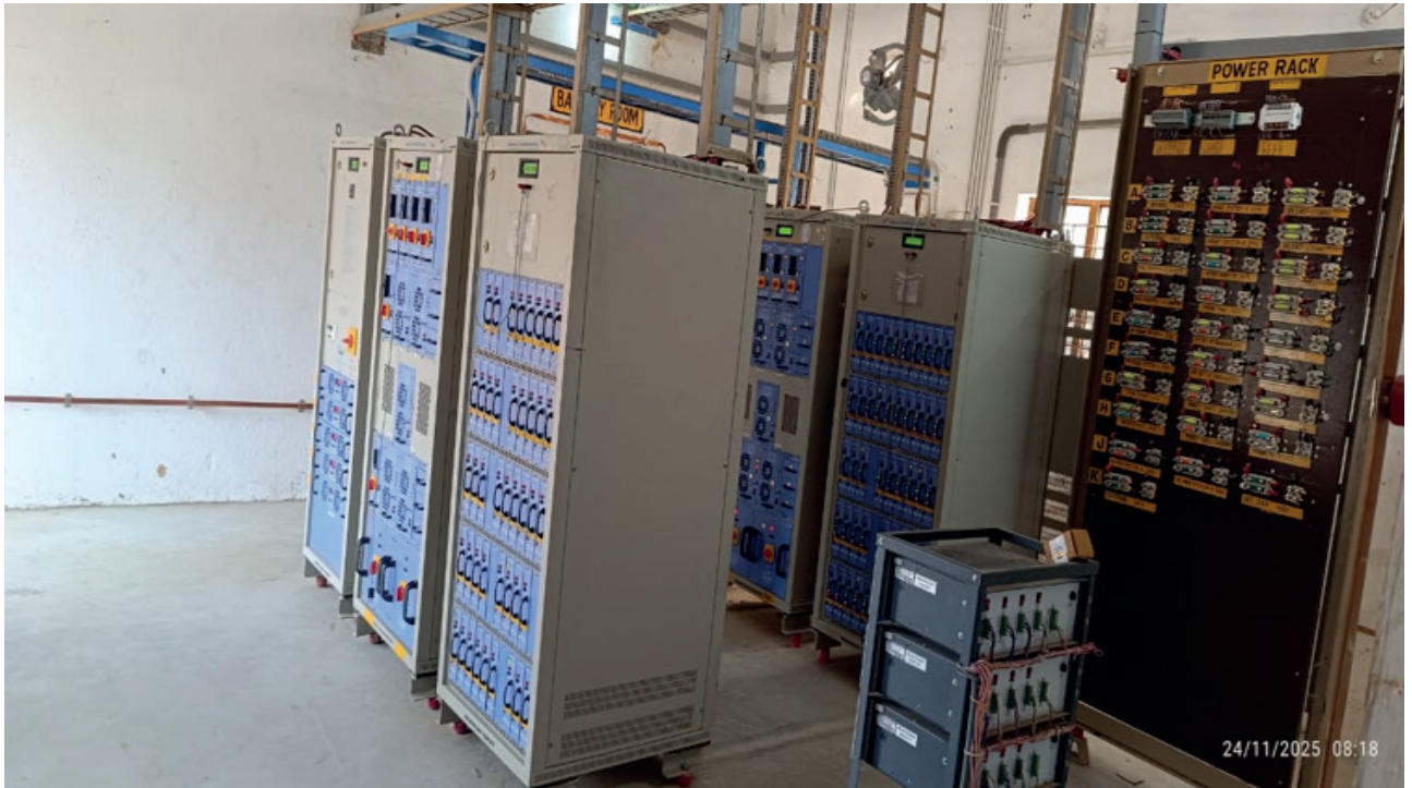
IPS ROOM AT KATHAUTIA STATION
